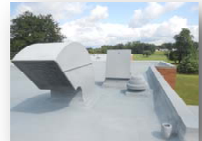
SPF ROOF SYSTEMS
